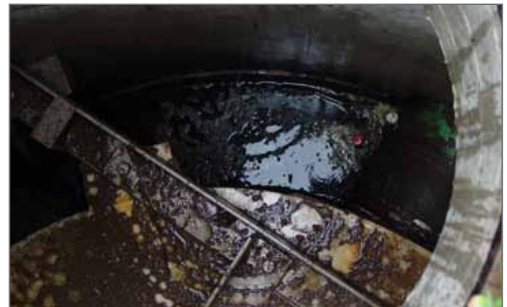
Fig. 8 View of outer annulus of floatables and oil collection zone.
