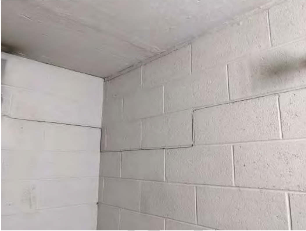
Photograph 7: Evidence of cracking and deterioration of stairwell
