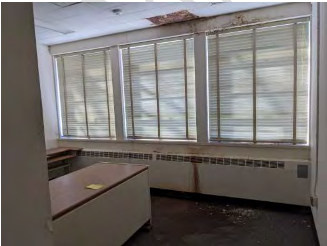
Photograph 15: Evidence of water damage (Building 3)
