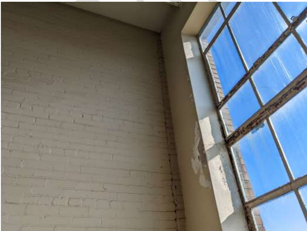
Photograph 6: Evidence of cracking and deterioration of stairwell
