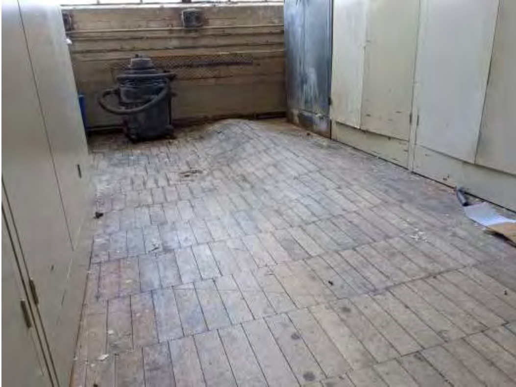
Photograph 16: Evidence of water damage and warped floorboards
