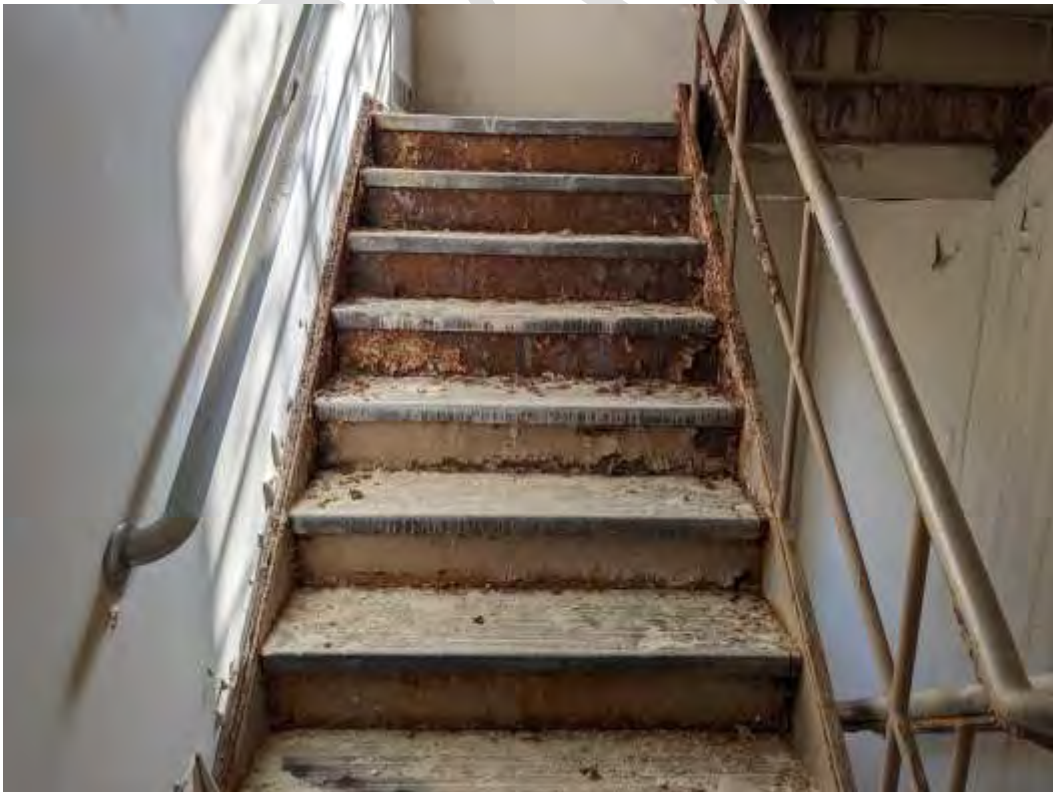
Photograph 12: Evidence of water damage (Building 3)
