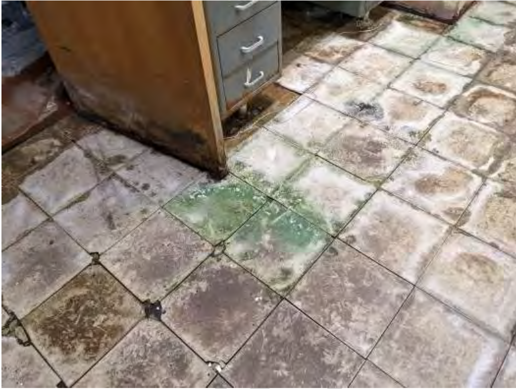
Photograph 11: Evidence of water damage (Building 4)
