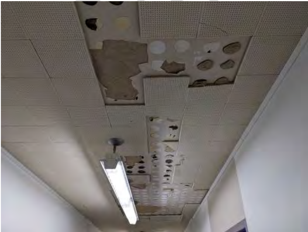
Photograph 10: Evidence of water damage
